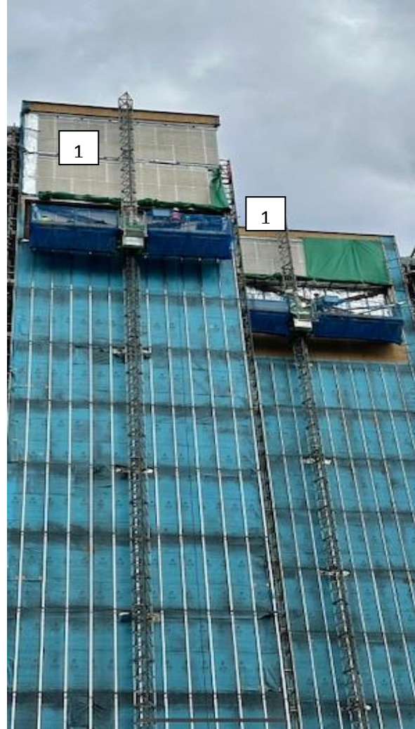
The above photo was taken 13/09/2023 and shows the progress of the works. Location 1 indicates the areas where all existing materials have been removed, and the new materials installed.
