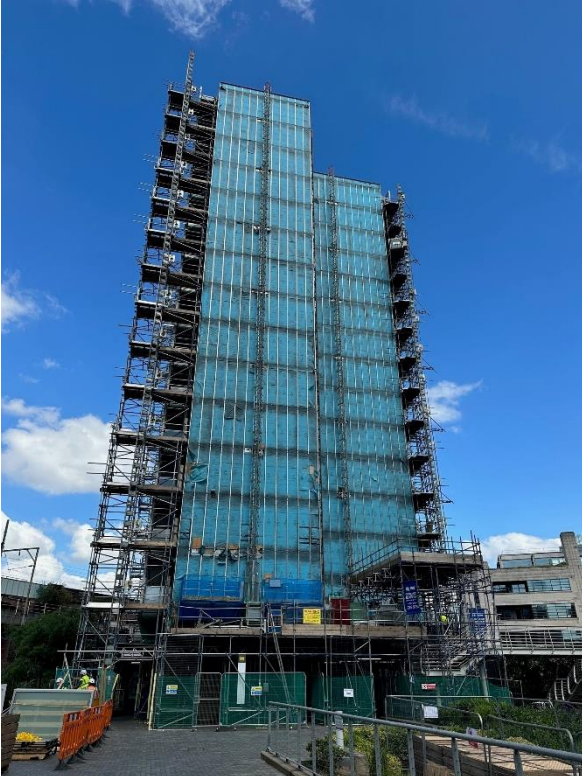
The above photo shows the South Elevation of Block 1 before removal works began. On this photo, the Terracotta Tile has been removed revealing the blue breather membrane.
