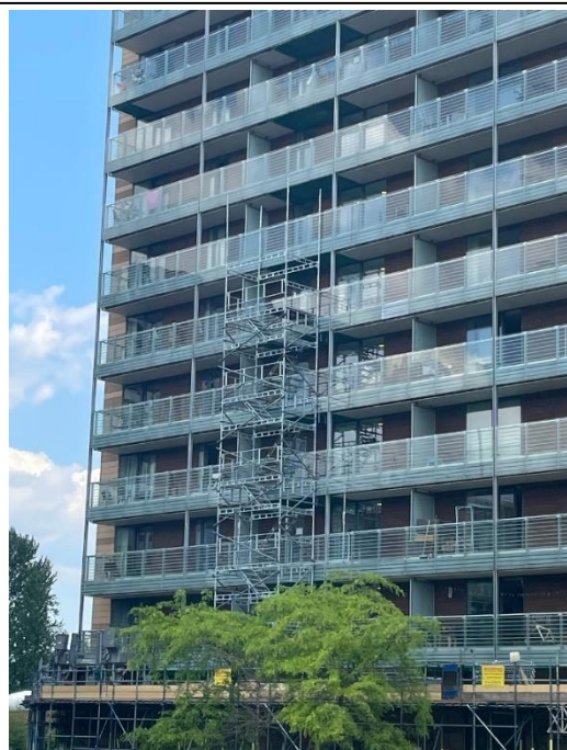
Block 1 – Installation of a Haki Staircase Haki staircases are required for the emergency exit of Operatives working on the balcony areas.
