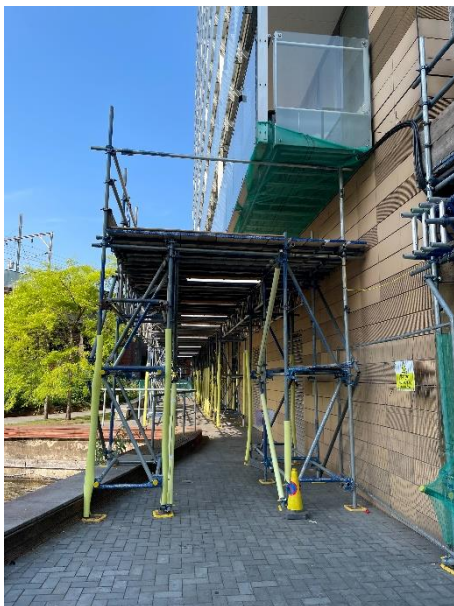
Block 1 – Installation of a Protected Walkway Scaffolding along the front entrance of Block 1 is for the protection of the public and will not be built any higher than the level shown in this photo. All access to the front entrance and emergency exit will be maintained throughout the work.
