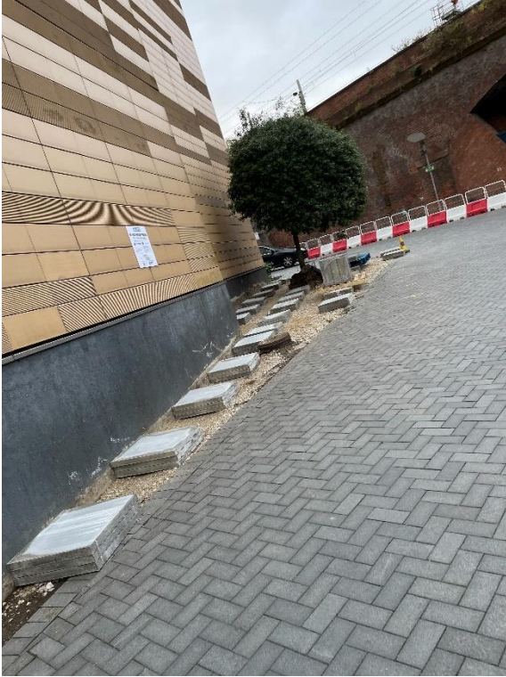
A photograph of the North elevation where the scaffolding will be installed.
